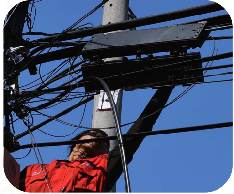
Telecommunication Network Infrastructure
